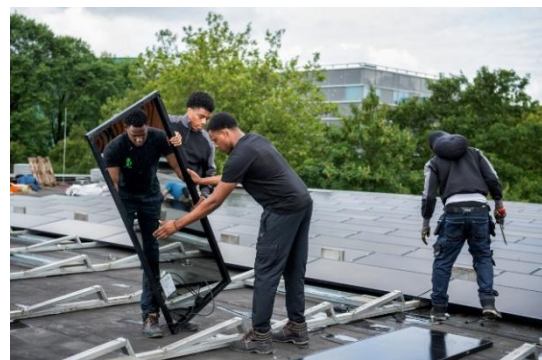
Figure 6: Second-hand solar panels installed at the Marineterrein by local installers from Southeast
